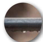
External Pipe Sweating
