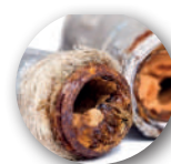
Internal Pipe Corrosion
